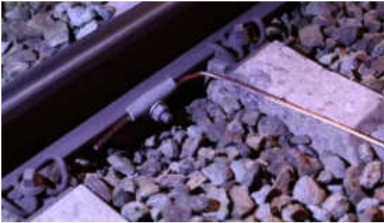
Abbildung 26: Experimental setup: copper cable firmly attached to one of the track rails.
